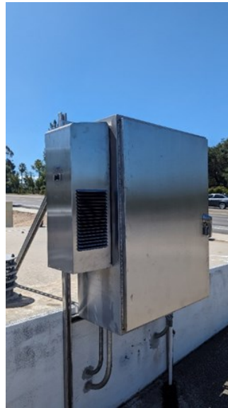
Figure 1 New Cabinet for RAM 3 Water Quality Panel Build
