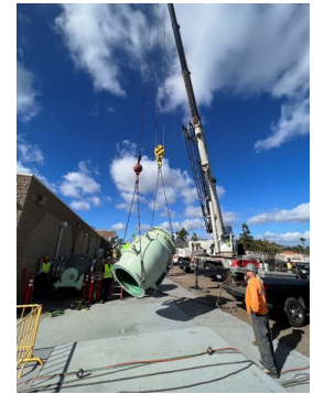
Flipping control valve on train 4
