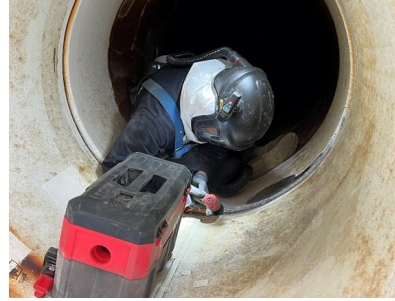
Staff removing rust and feathering the existing coating prior to application of new epoxy lining
