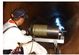
The AFO System was installed in Pipeline 4 in 2009
