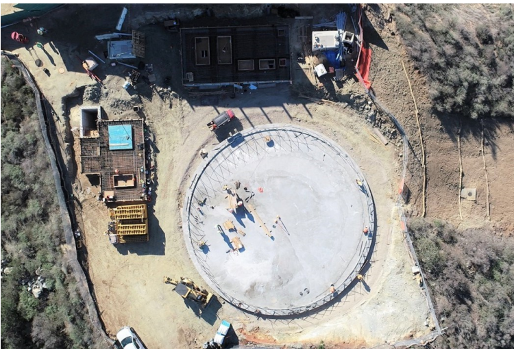
Reservoir Floor (Center), Flow Control Facility (Left), and Valve Vault (Top)
