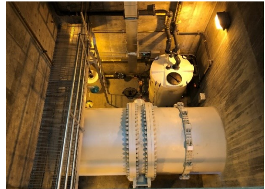
72-inch Inlet Pipe and 500 Gallon Chemical Storage Tank
