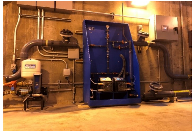
Dual Chemical Feed Pump Skid
