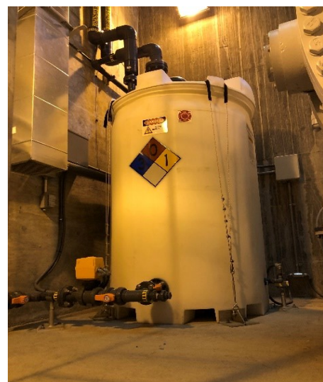
500 Gallon Chemical Storage Tank
