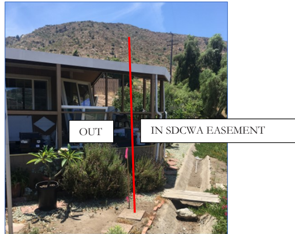
Deck and awning (before removal). Pink flag on stake is east edge of Second Aqueduct easement
