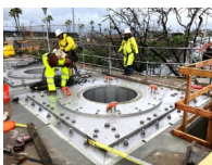
Figure 2: Pump Installed in Vault
