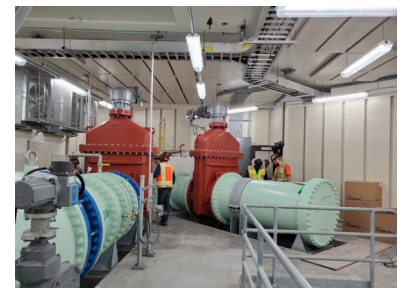
San Diego 28 Flow Control Facility – Interior of New Facility
