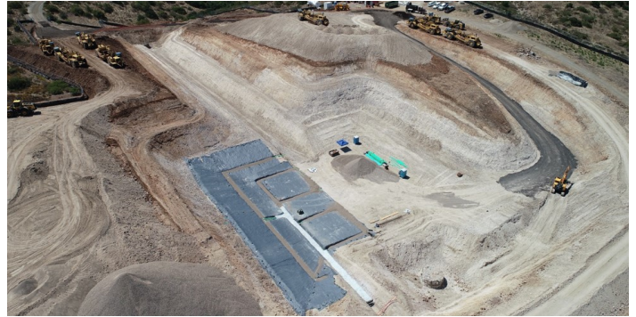
Drone photo of mass excavation and tank subgrade preparation for FRS II
