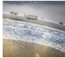
Figure 2 - Weeping Defective Welds
