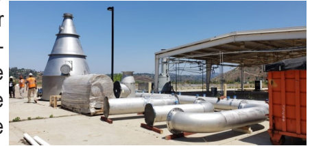
Speece Cone, Discharge Ports in the Foreground Pass
