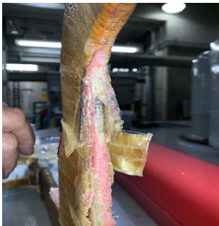
Insulation damage on a removed bus bar
